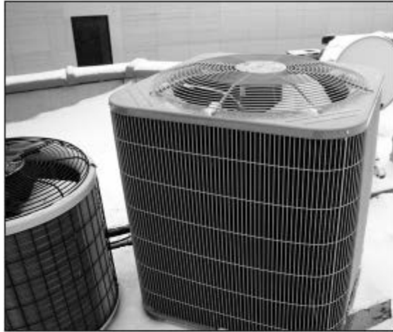
Air conditioning systems
